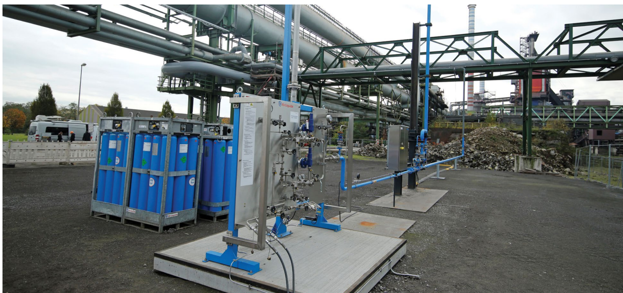
Air Liquide Testing facilities for a new blast furnace process involving hydrogen are seen at a ThyssenKrupp steel factory in Duisburg, Germany, in November 2019. REUTERS/Leon Kuegeler.
