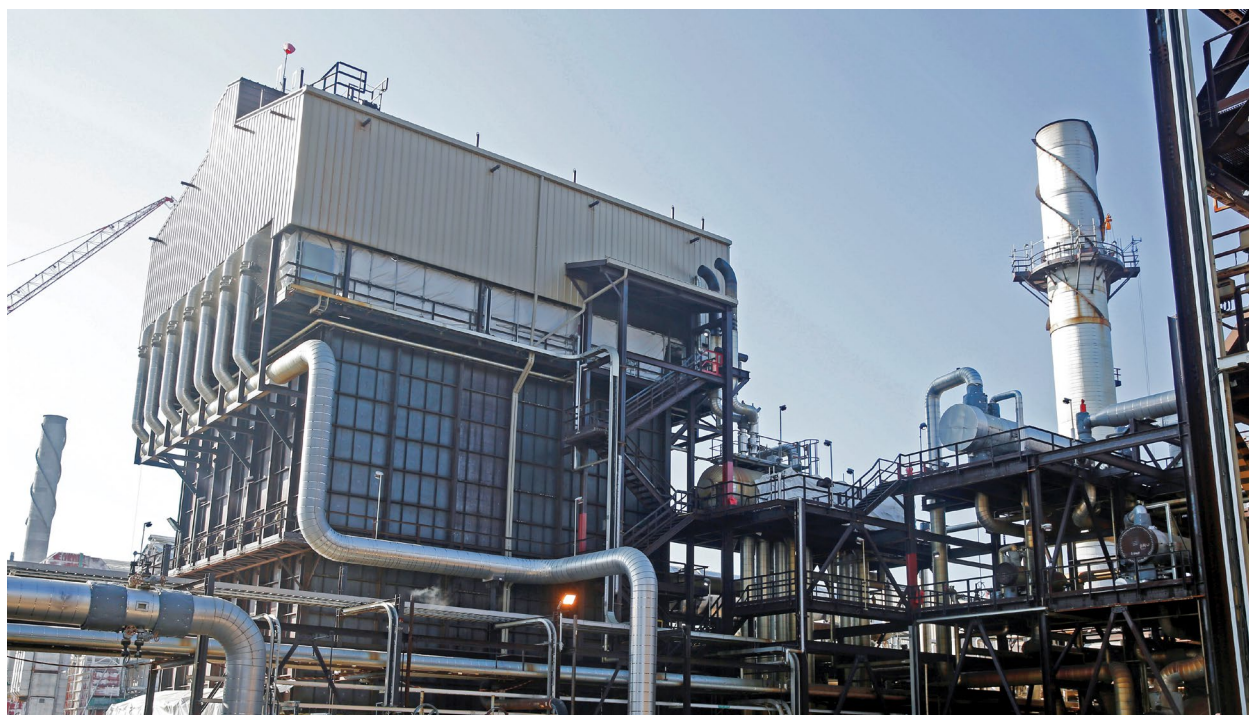
Pipes run through Shell's new Quest Carbon Capture and Storage facility in Fort Saskatchewan, Alberta, in October 2021. REUTERS/Todd Korol.
