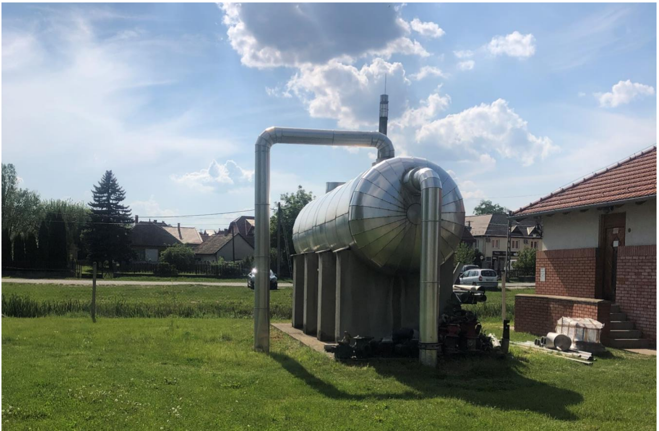
Geothermal water well in Veresegyház, Hungary
