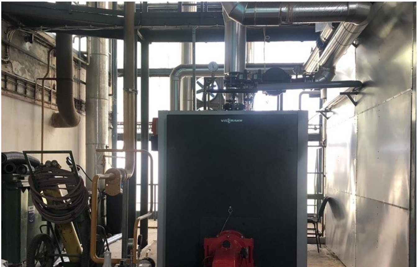
Geothermal water plant in Szeged, Hungary with new, more efficient radiators for local residences
