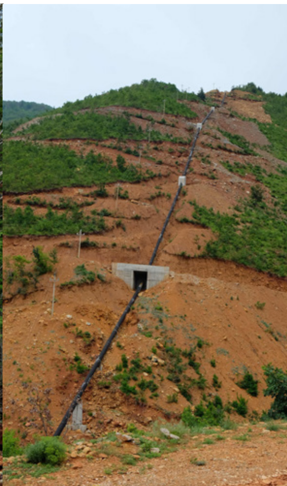
Figure 17: Erosion around the penstock
