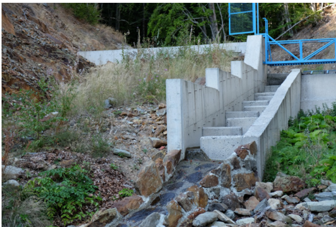
Figure 6: An almost dry fish pass at the Brajcinska reka 1 intake
